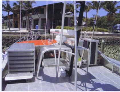
Rooftop power and air con
